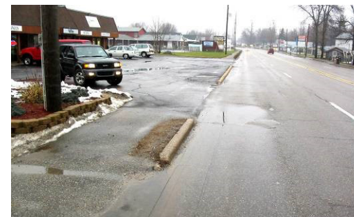
poor driveway definition
