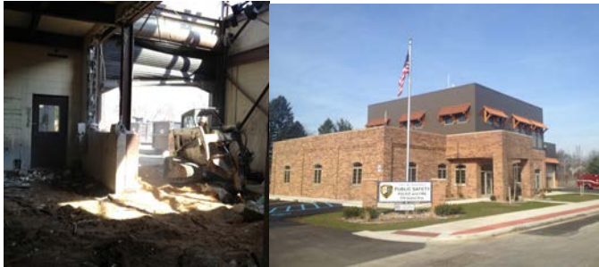
Renovation and adaptive reuse of the former dewatering facility took less than a year. The city's new public safety building opened in December 2012.
