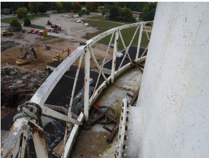
12) The balcony is in fair condition. The coating is in poor condition.
