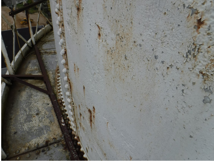
16) The sidewall is in good condition overall. The coating is in poor condition.
